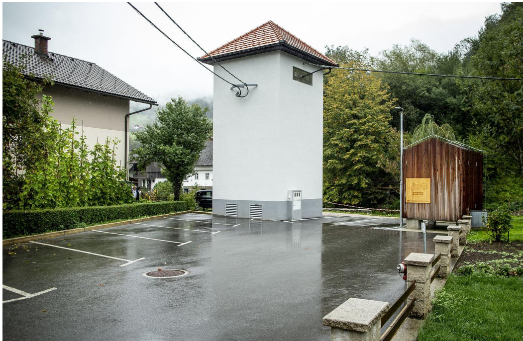
Figure 4: Transformer station (left) and system battery (right).
